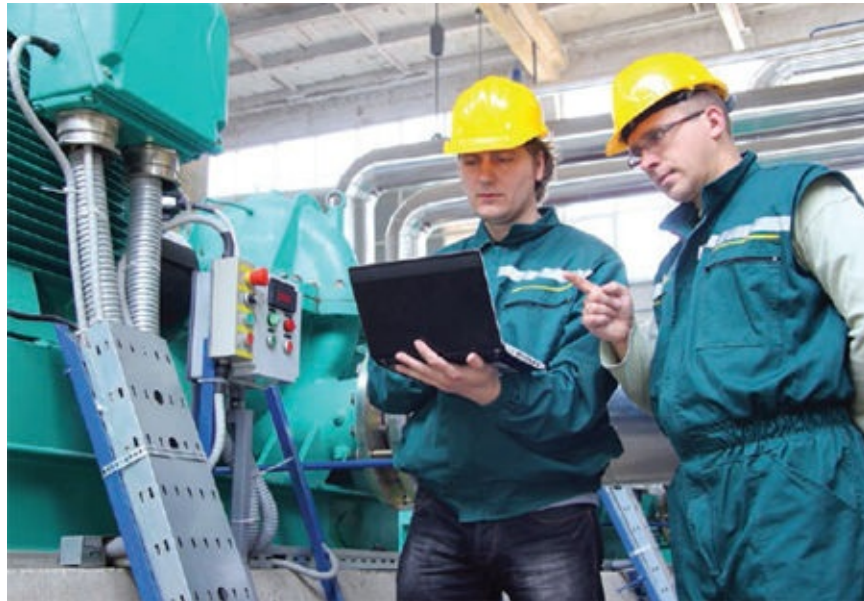
Figure 9.9 Scheduled maintenance checks at a power plant
